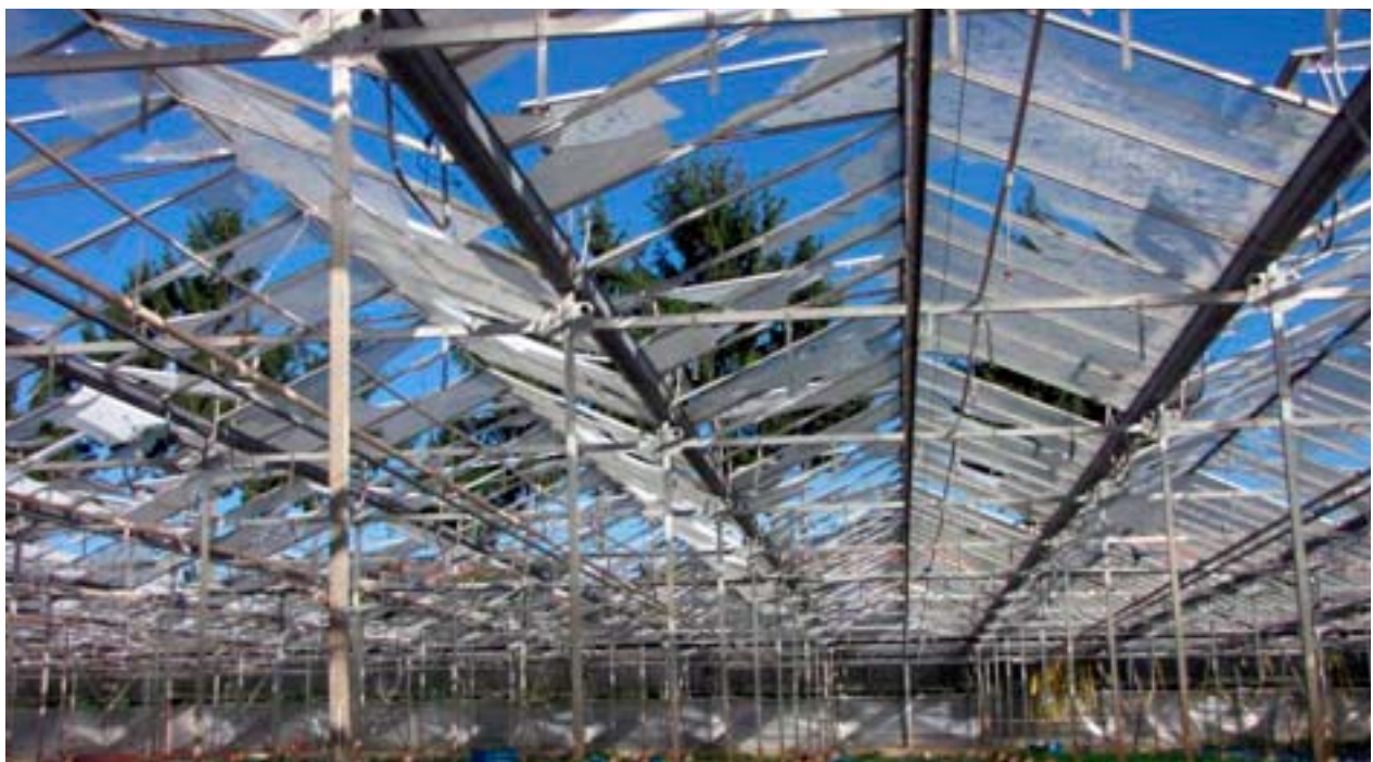
Figure 8: Hail damage to a large greenhouse
