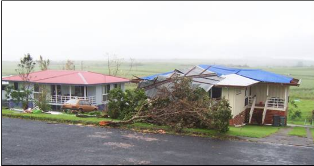
Figure 2: Roof damage in Hudson
