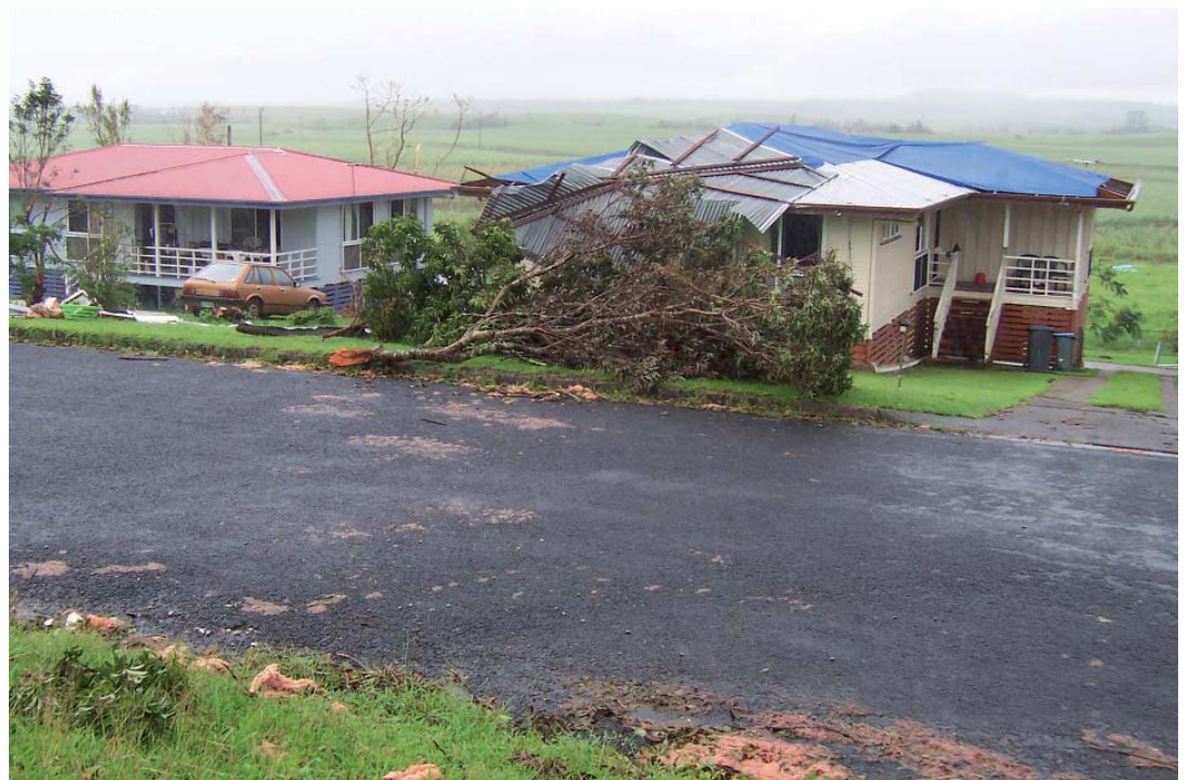
FIGURE 8: ROOF DAMAGE IN HUDSON
