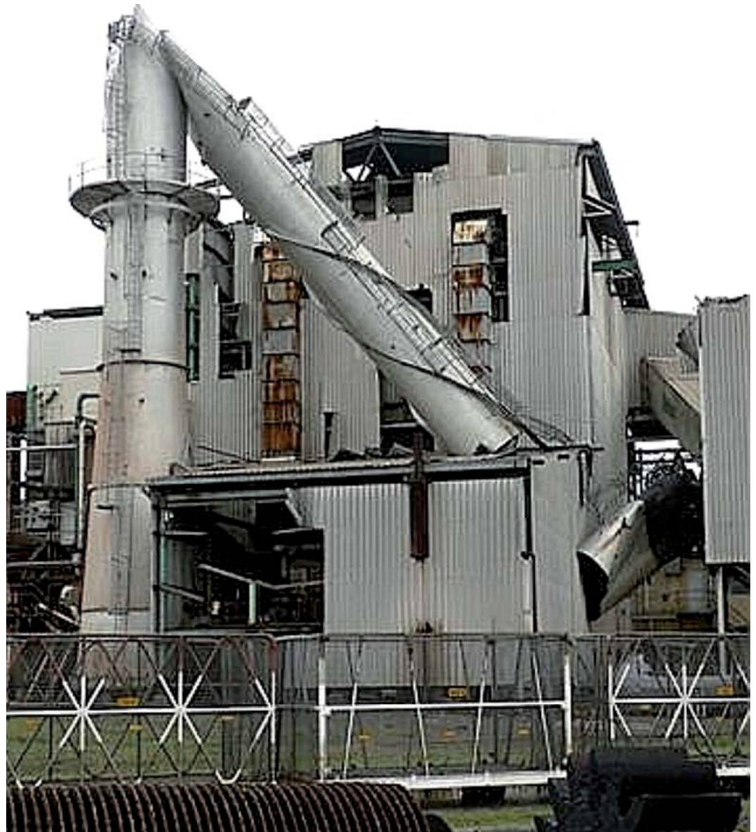
FIGURE 6: INDUSTRIAL DAMAGE AT MOURILYAN MILL, MOURILYAN
